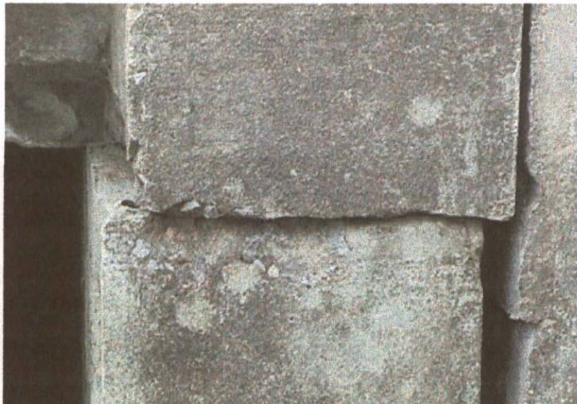
CRACK AT BACKWALL ABUTMENT #1 WITH MISALIGNMENT
