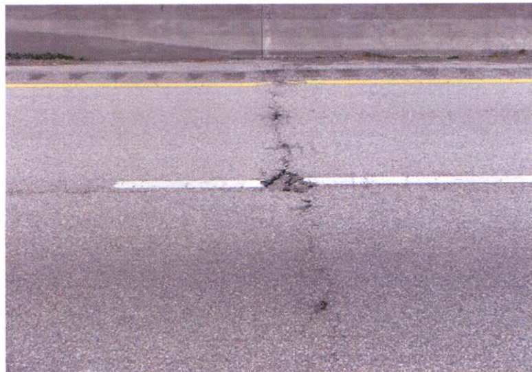
POTHOLE @ B-APPR JOINT
