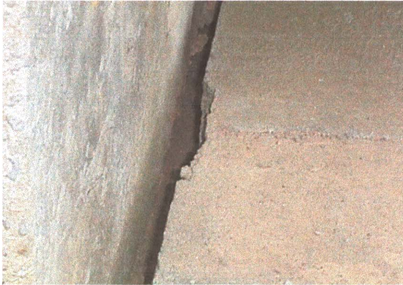
SETTLEMENT ABUTMENT #2 & SEPARATION OF SLOPE PAVEMENT
