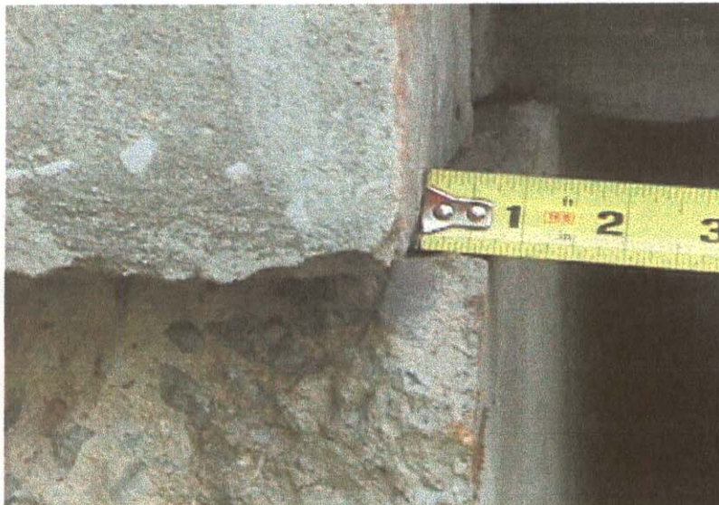
CRACK AT BACKWALL ABUTMENT #1 RIGHT SIDE WITH MISALIGNMENT
