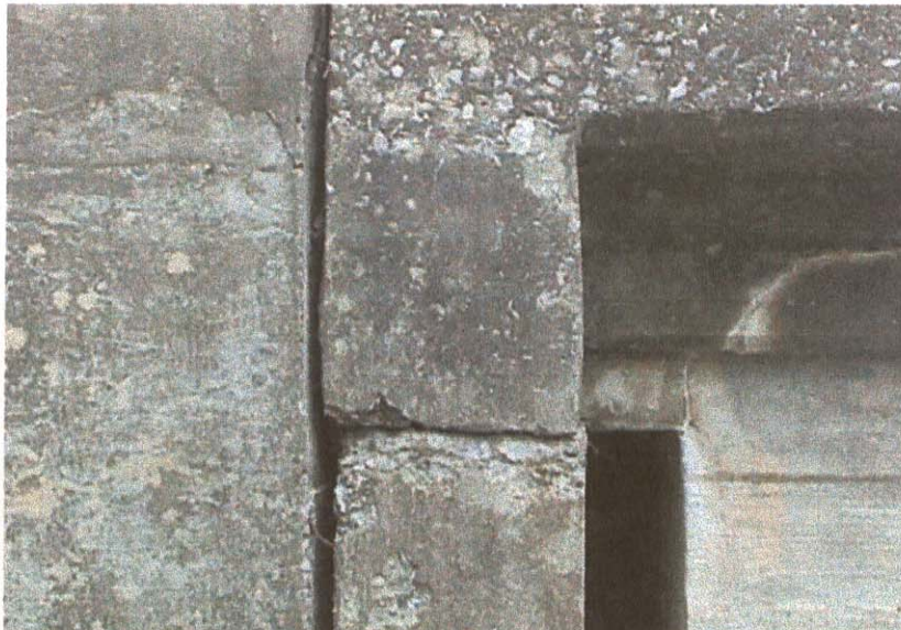
CRACK AT BACKWALL ABUTMENT #2 WITH MISALIGNMENT
