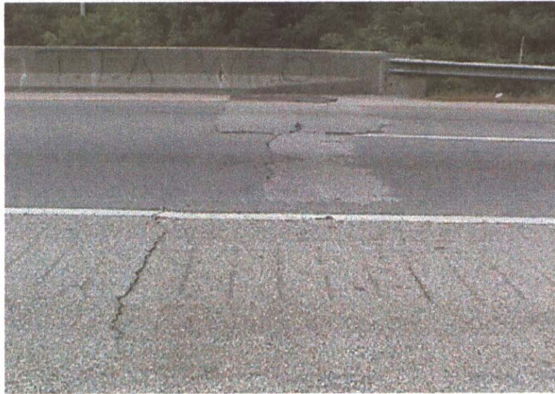
APPROACH 'A' SETTLEMENT
